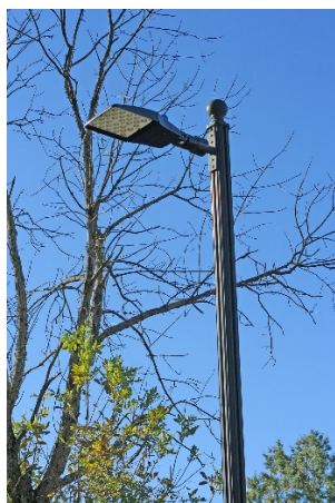
Example of Mongoose Light pole: Will be LED and some Amber Bulb (close to Ocean) the shape of these lights is in compliance with the COJB Turtle Ordinance
