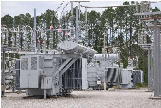
Aging autotransformer (foreground); new autotransformer (middle ground)
