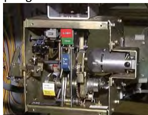
Spring mechanism breaker
