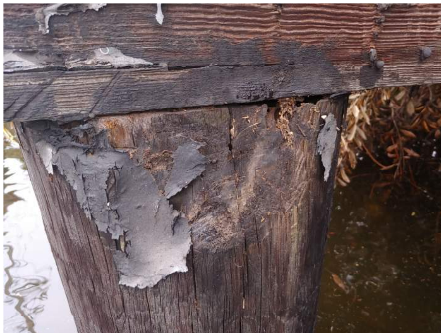
Photograph #2 Deteriorated Top of Pile North Bent
