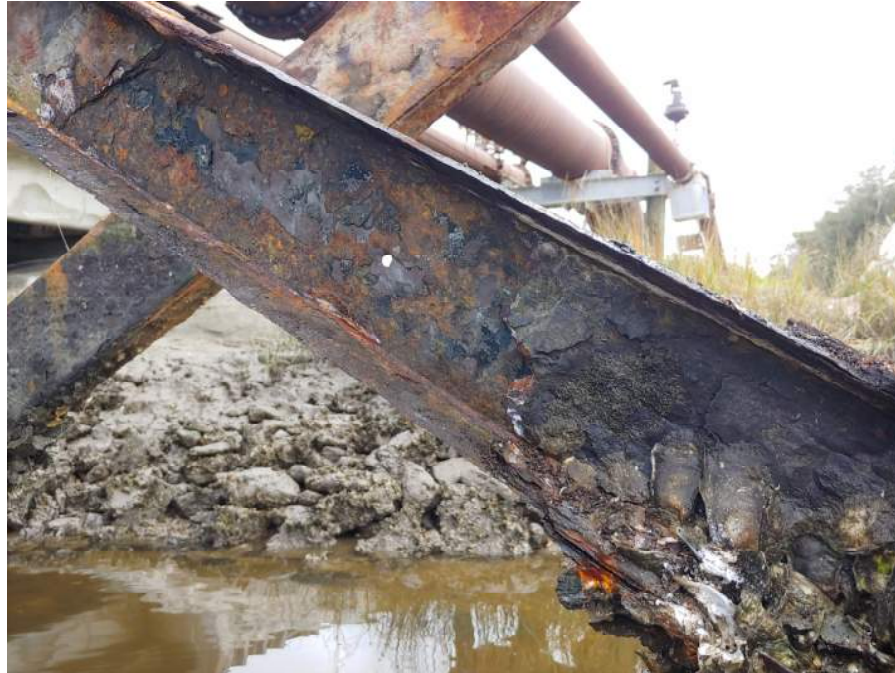
Photograph #21 Typical Corroded Cross Bracing
