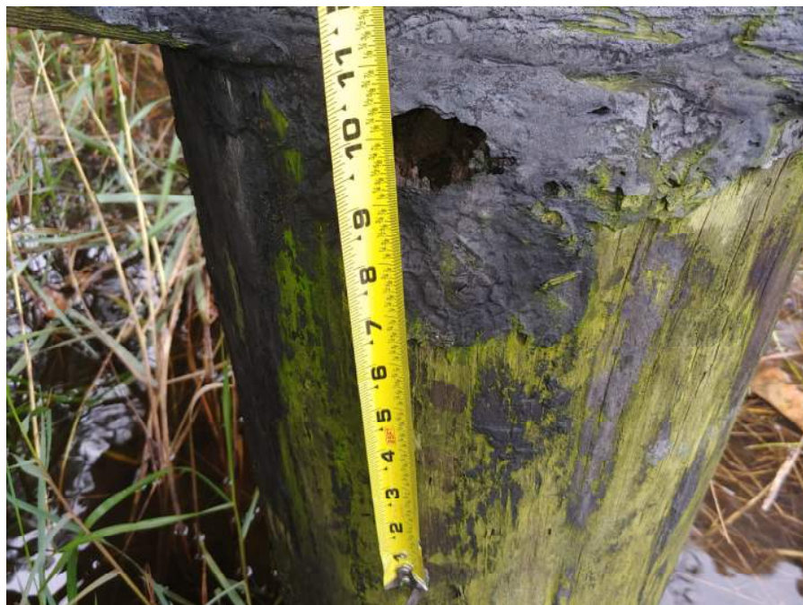
Photograph #6 Deteriorated Pile South Bent
