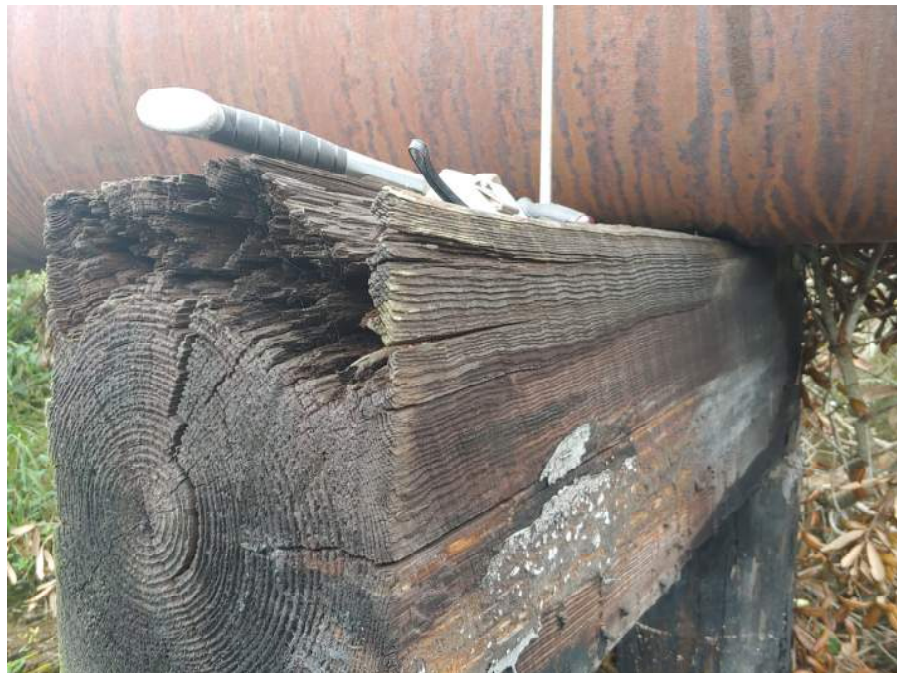
Photograph #4 Rotted Beam North Bent
