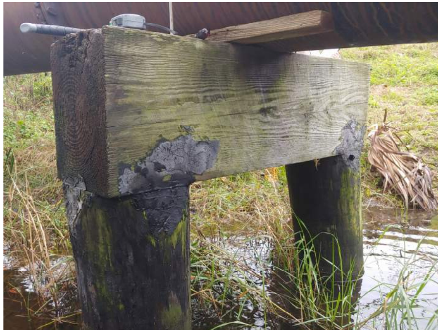
Photograph #5 End of Beam Deteriorated South Bent
