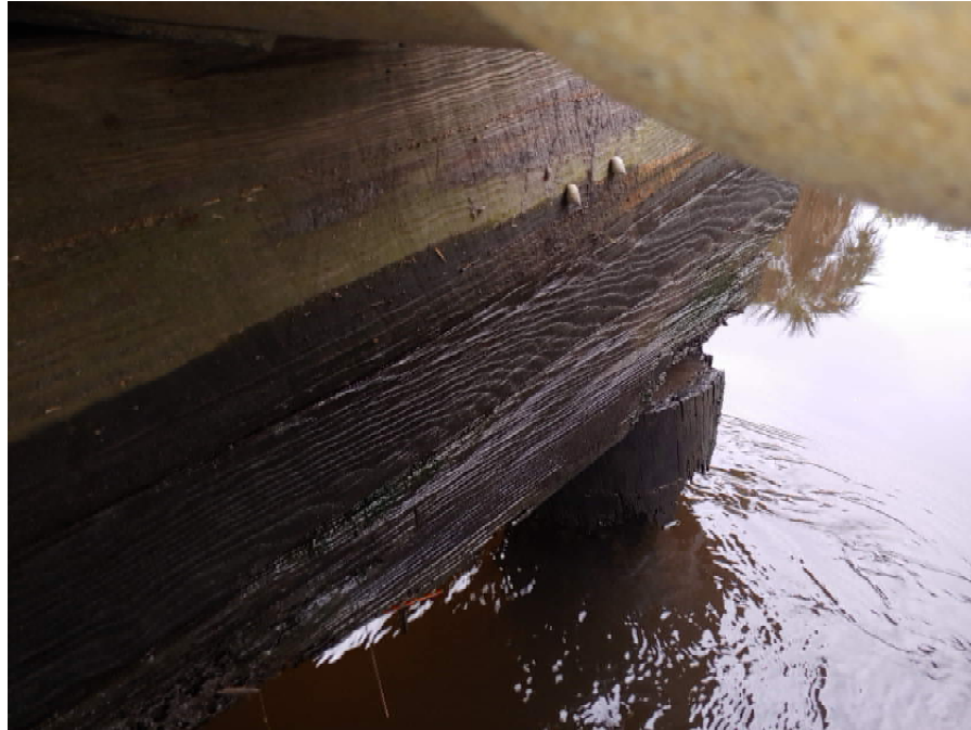
Photograph #9 Rotted Pile and Beam South Bent
