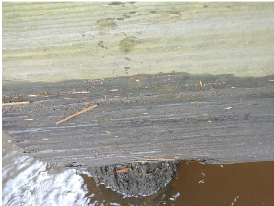
Photograph #8 Rotted Pile and Beam North Bent
