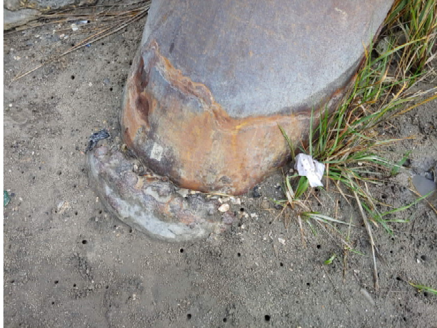
Photograph #13 Exterior Corrosion of 24" Pipe
