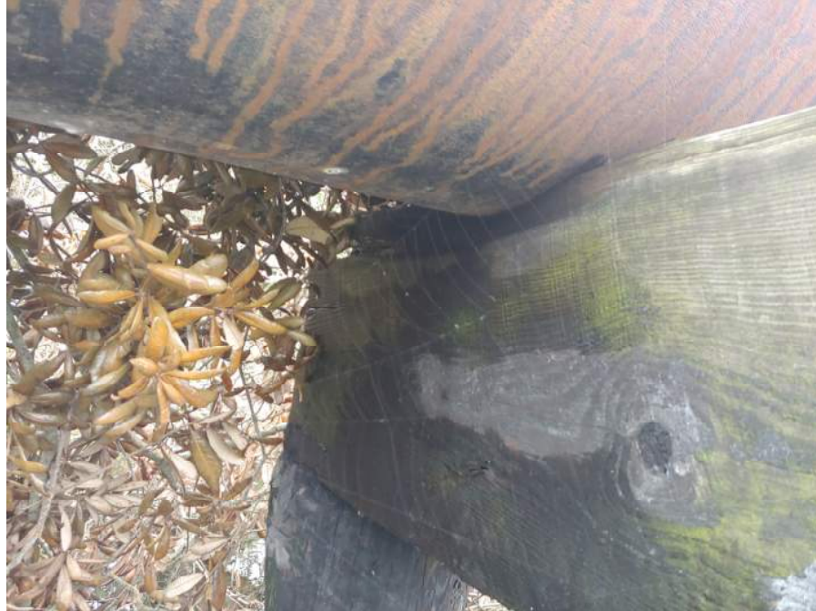
Photograph #3 Pipe Crushing Top Beam North Bent
