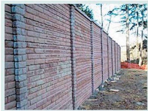
Example of an inappropriate solid brick wall.
