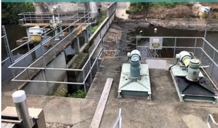
South Beach Basin Pump Station looking north
