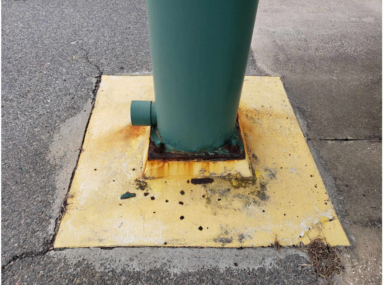
Southernmost Column Support Rust
