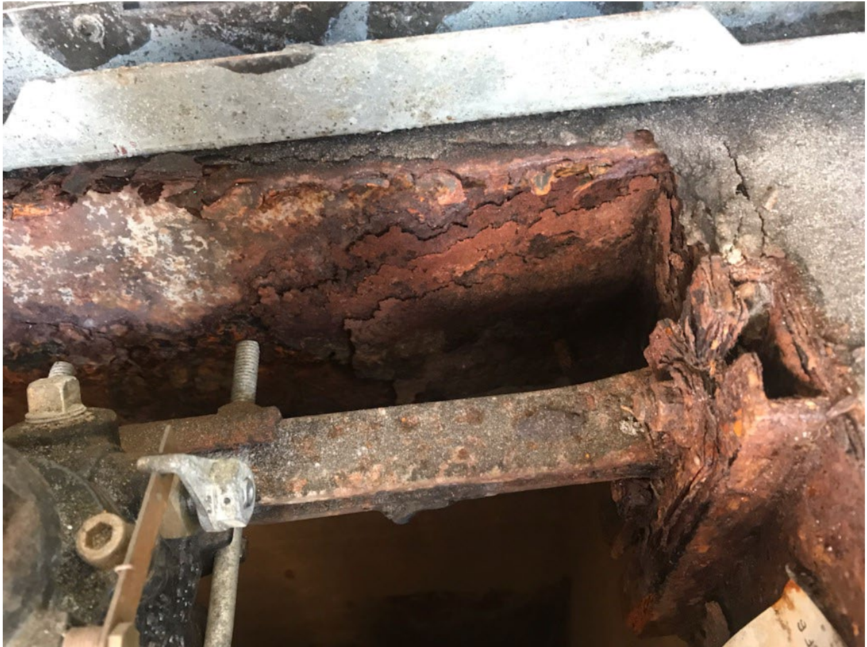
Southernmost Pump Vault Rust
