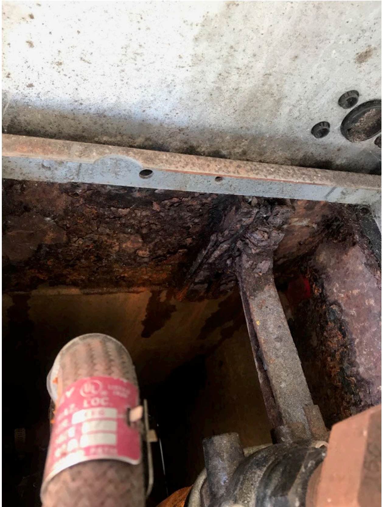
Southernmost Pump Vault Rust
