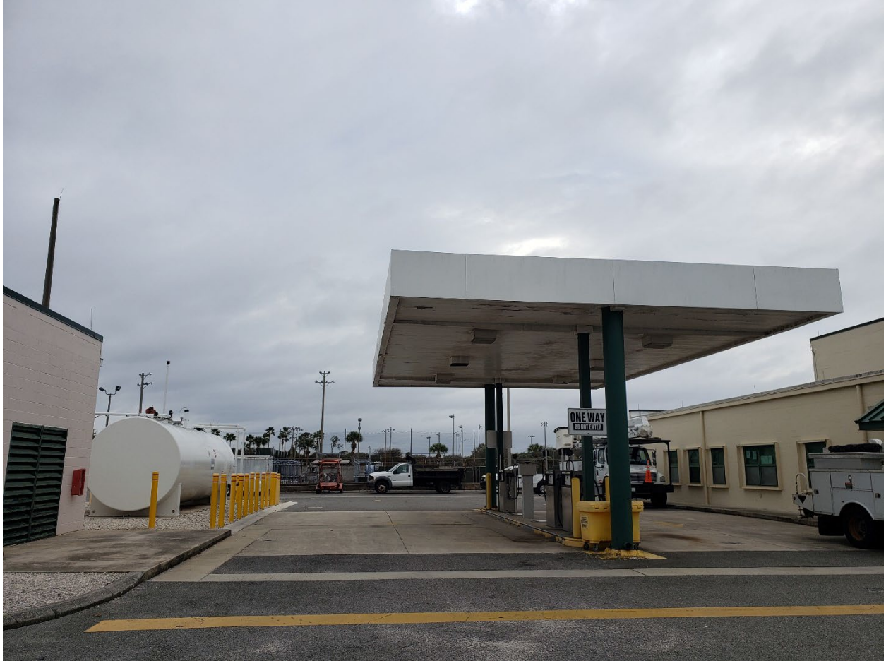
O&M Fuel Pumps and Canopy
